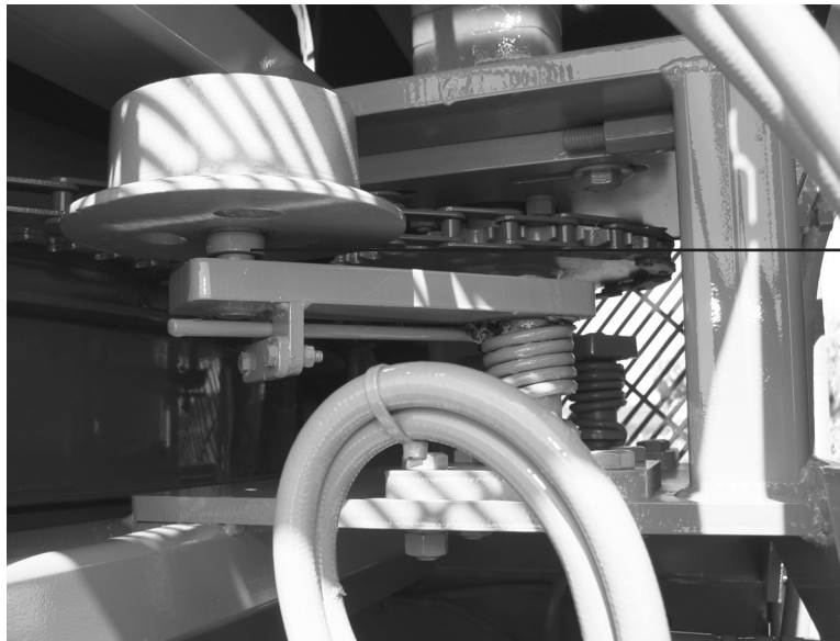
tub chain idler pivot lubrication point (Ref #2)
