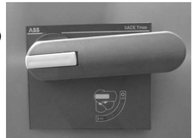
Figure 3 Main Breaker (Shown in the OFF position.)
