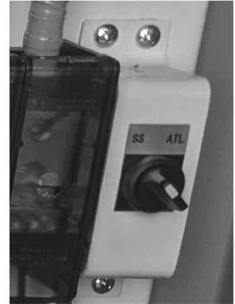
Figure 2 SS/ATL Switch (Inside Control Panel.)
