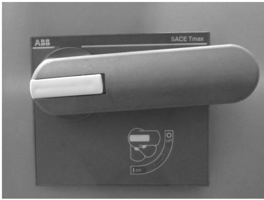
Figure 3 Main Breaker (Shown in the OFF position.)
