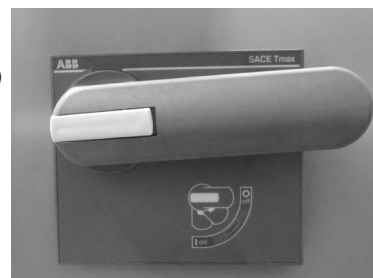
Figure 3 Main Breaker (Shown in the OFF position.)
