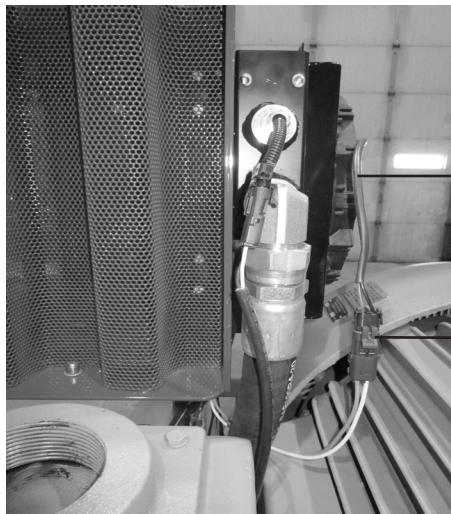
Figure 13 Disconnect fan from fan controller
